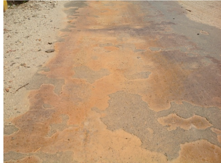
slight deck deformation on running path
